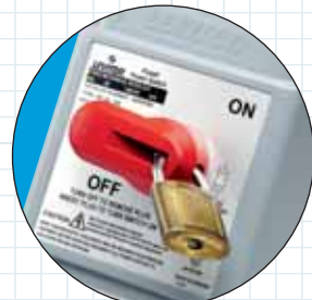
Handle with padlock installed
