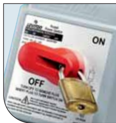
Handle with padlock installed
