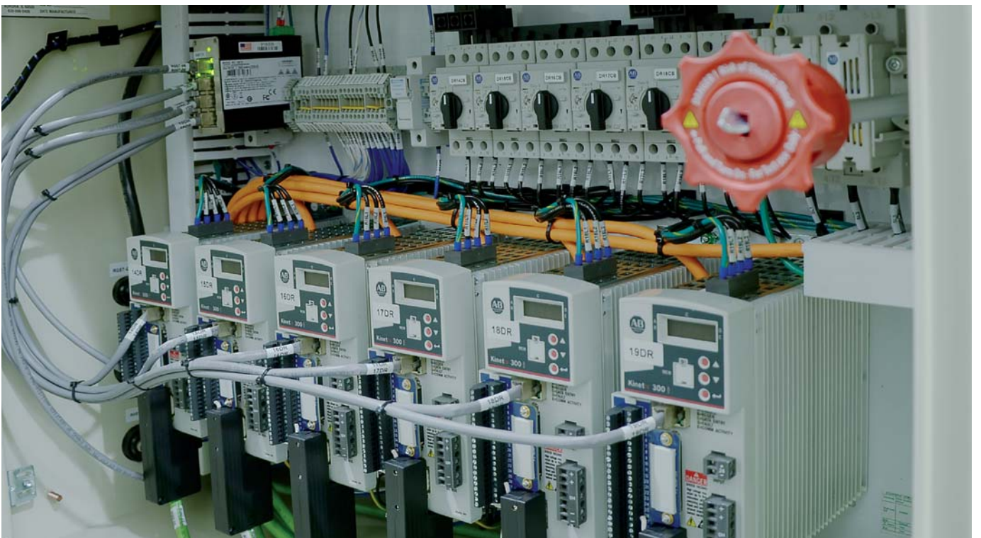
Wiring inside and on the cabinet: LUTZE cable assemblies are always system compatible and offer great flexibility.
