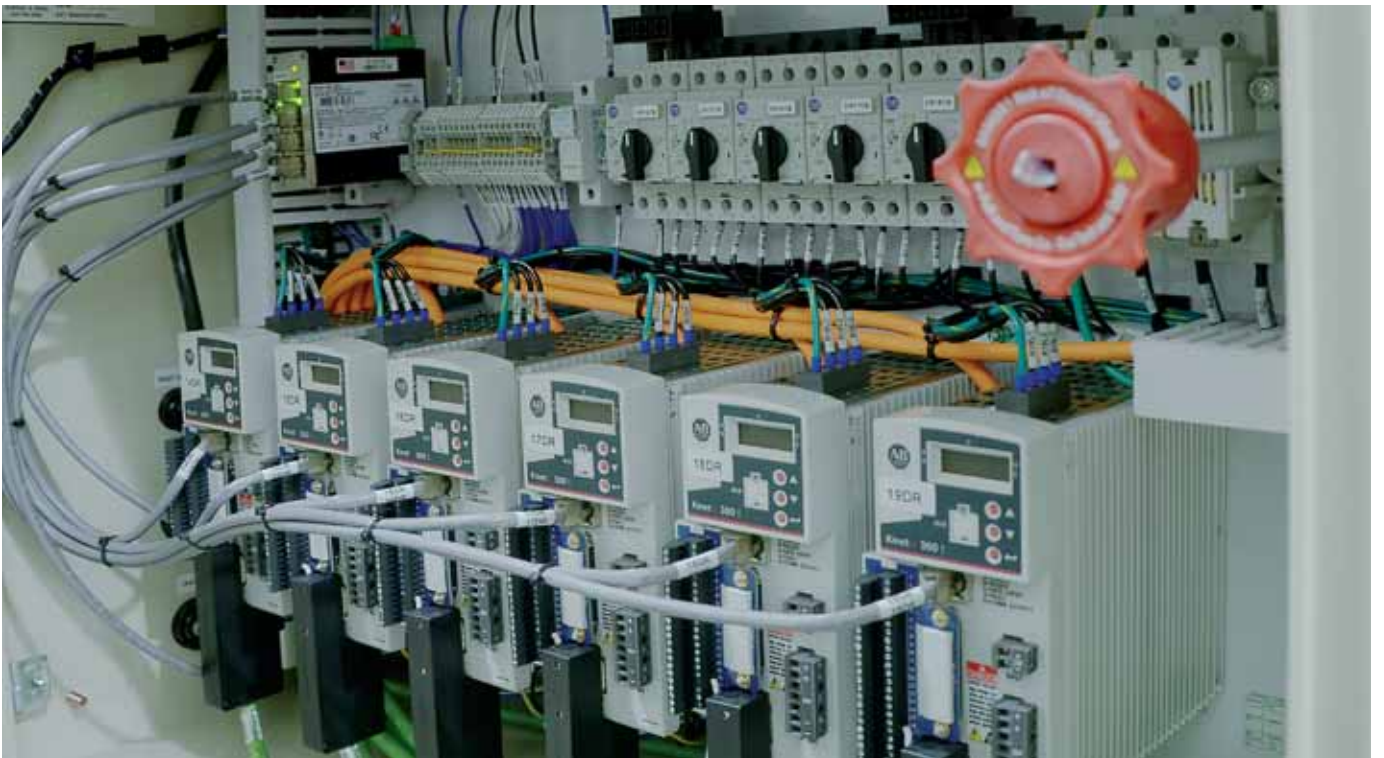
Wiring inside and on the cabinet: LUTZE cable assemblies are always system compatible and offer great flexibility.
