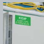
Control Panel Labeling
