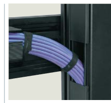
4 horizontal cable management
