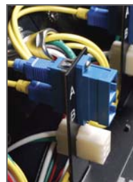
Internal SC and electrical breakout
