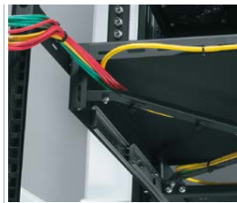
articulating cable arm keeps wires from getting pinched when the drawer is pulled open or closed shut
