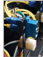
Internal SC and Electrical Breakout
