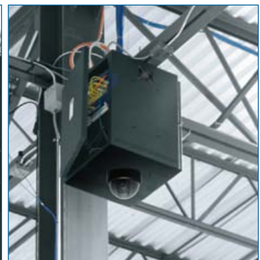
a typical warehouse IDF installation with optional dome camera mounted underneath
