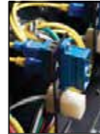
Internal SC and Electrical Breakout
