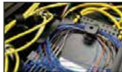
Internal Fusion Splice Tray with Cable Management
