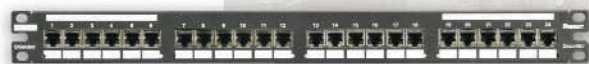
24-port, flat modular patch panel, populated with pre-terminated shielded cassettes with shielded jack modules.
