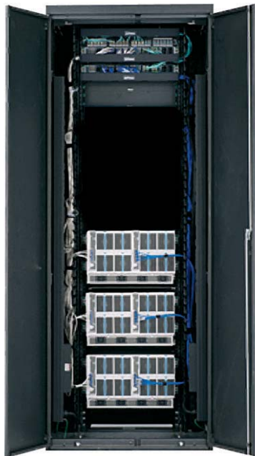
(32" Cisco^ UCS Pre-Configured Physical Infrastructure shown in a Net-Access™ Cabinet)
