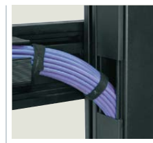
4 horizontal cable management
