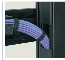
4 horizontal cable management
