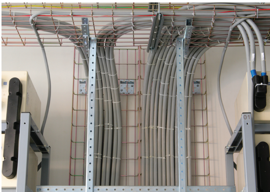
▲ Cloth cable installed in a Central Office.
