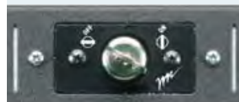
Remote Power Switch
