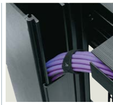
3 generous hidden vertical cable management
